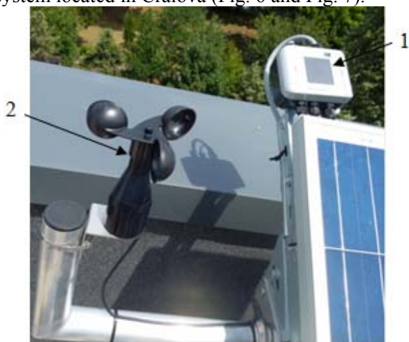
Fig. 6. Equipment for measuring weather parameters: 1- pyranometer; 2- anemometer.
