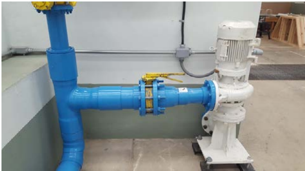
Fig. 4. Centrifugal and submersible pumps.
