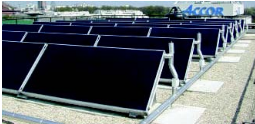
Fig.15 Solar collectors mounted on the roof of thermal station.
