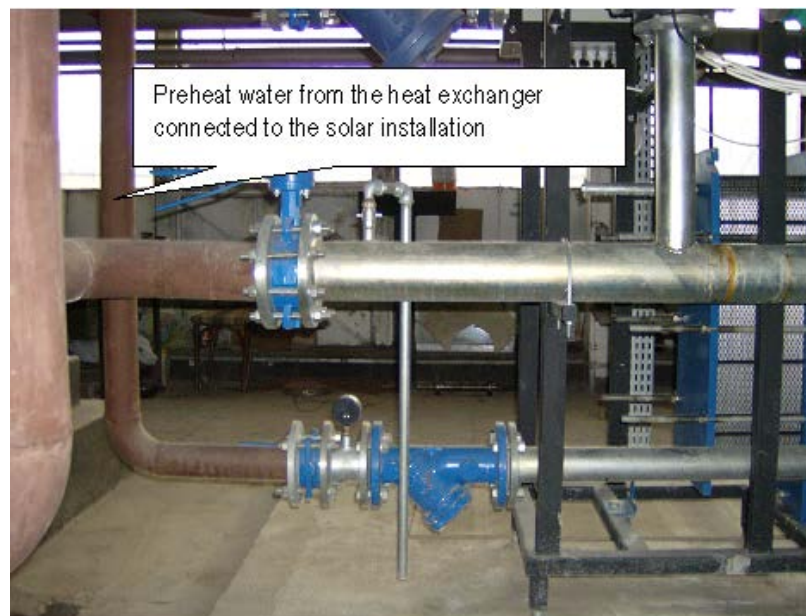
Fig.13 Zone of connection with the piping from the solar collectors.
