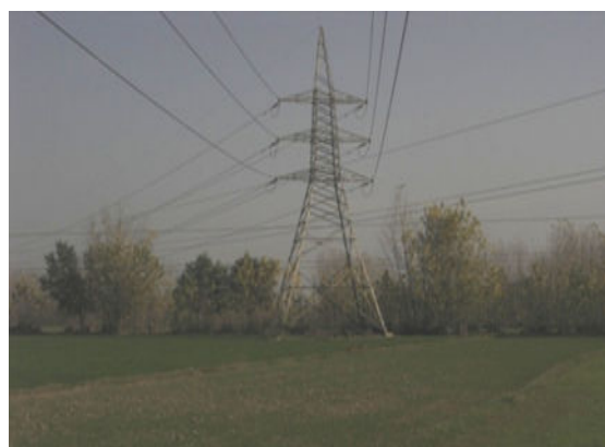
Figure 1. Overhead Electric Power Line
