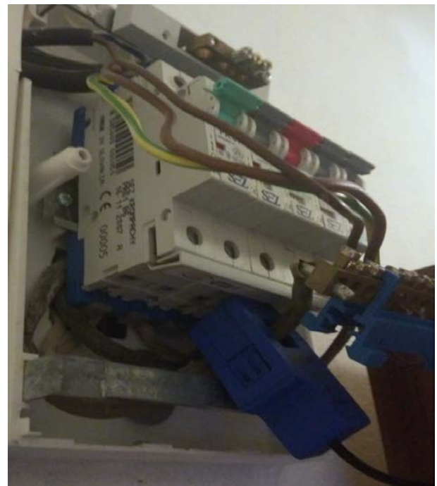
Fig.7 Sensor deployment on flat house phase wire
