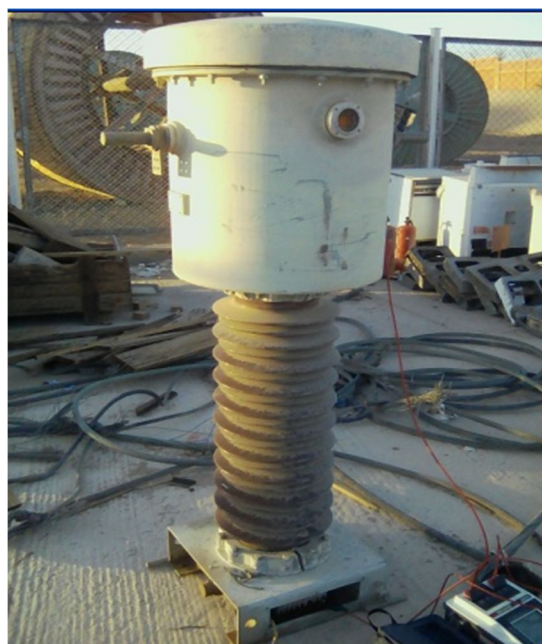
Figure 1: The current transformer was used.
