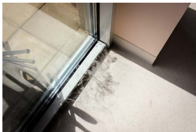
Fig. 13 Sub-pressure conditions, in connection with spot caused smoke on the outside of the building allowed to detect leakages by the observer in the inside. Here: air leakage at the lower edge of the glazed façade
