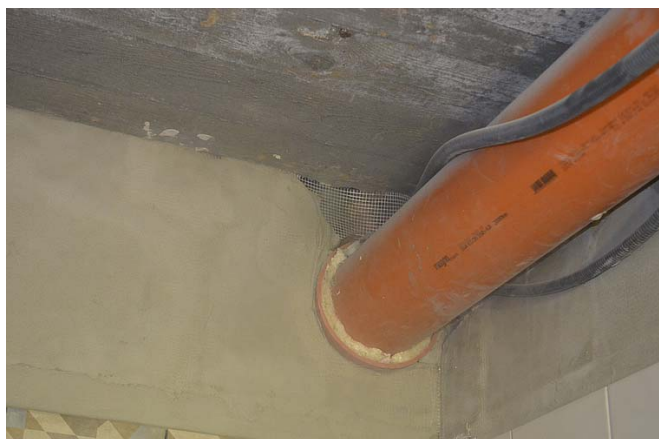
Fig. 11 Leakage caused by improper finishing of the sewage installation cut through the partition [author's own source]
