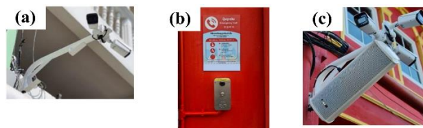
Fig. 2. Primary components of intelligent surveillance system: (a) security camera, (b) emergency hotline station, and (c) smart public announcement speaker
